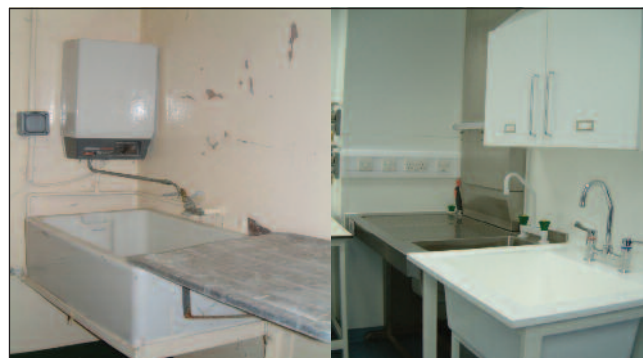
Figure 5. (Left) Peeling paint, poor design and surfaces that can harbour pathogens are unlikely to be encountered in establishments today. If the fabric of designated rooms deteriorates the room would be either removed from the schedules on the Certificate of Designation or refurbished. (Right) modern facilities are built to a high specification making cleaning and maintenance easy.
